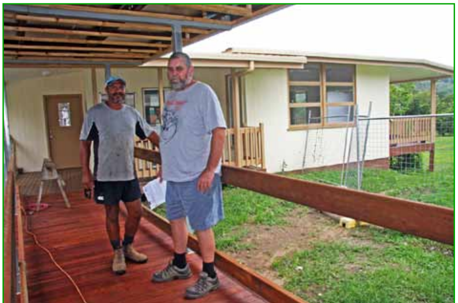
Carpenter Patrick Nandy and Housing Coordinator Mark Zippel discussing the finishing touches to a walkway between the new training rooms and Council Chambers
