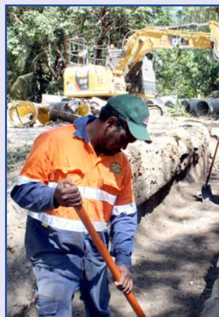
Culvert repair and roadworks on the road to Wungu is expected to be finished within the month thanks to Yarrabah Shire Council.
